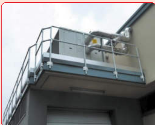
116 • Example of guardrail mounted on a building
